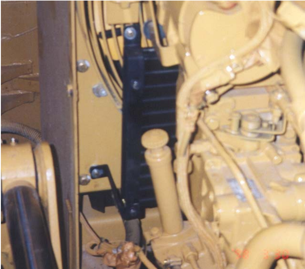
Left side of condenser assembly.
